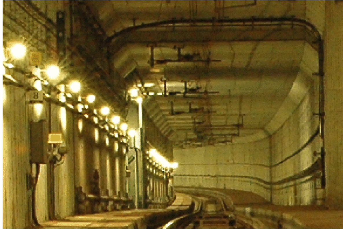
PHOTO 1 IMPACTING ON THE TRACK CENTRE INSIDE THE TUNNEL AT DOWNTRACK CH64.063 OF THE MTRC TSEUN KWAN O LINE
